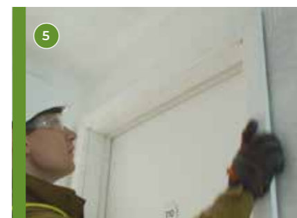
5 Fit the pre-cut door stops and then assemble, using the Hoffman fittings, the pre-mitred architrave and fit to the frame.
