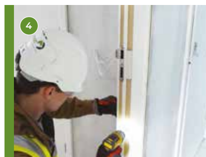
4 Secure the doorset to the structural opening, seal the gap between the structural opening and frame if a fire door to BS8214:2016.
